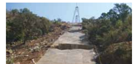
Anchoring a reno mattress along the RoW, with a cable crane in the background.
