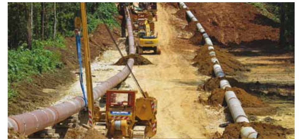
Welded pipe for the PNG LNG Pipeline ready to be lowered in.
